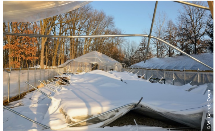
Figure 1. Heavy, wet snow accumulation on the double-poly greenhouse resulted in collapse of the greenhouse structure. Photo by W. Garrett Owen.
