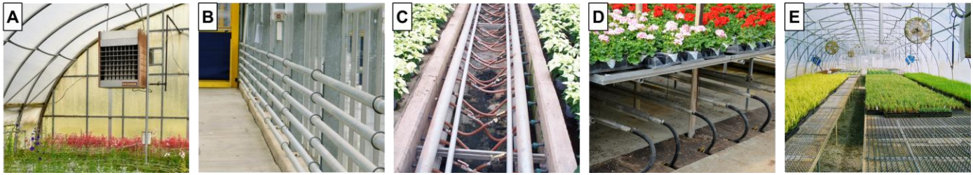
FIGURE 13. In greenhouses, (A) overhead unit heaters, (B) perimeter, (C) radiant floor, (D) under-bench, and (E) bench-top systems can be used independently or together to manage the air temperature in the growing environment.
