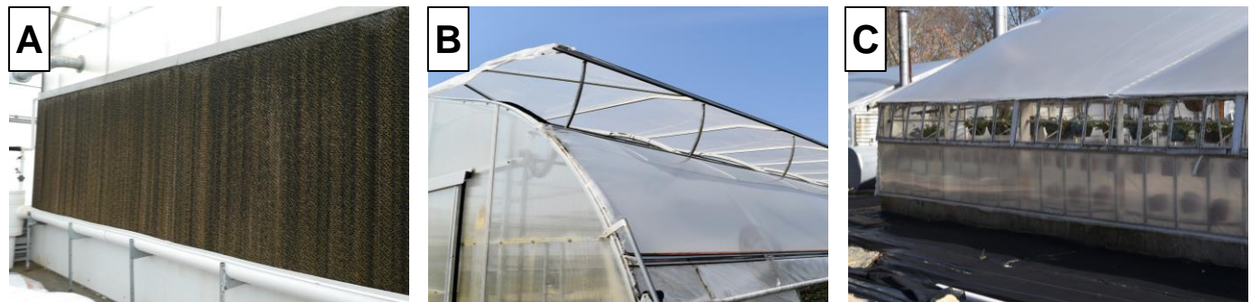
FIGURE 15. To cool greenhouses, (A) evaporative cooling systems, (B) ridge, and (C) eave vents can be installed.
